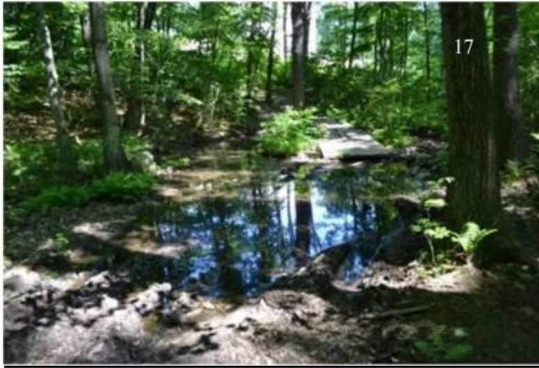
Moose Pond Town Forest - Complete trail failure and wetland violation caused by OHRVs; bridge had to be removed and trail re-routed.
